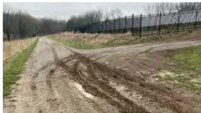
Current Roadway Condition Following Rainfall
